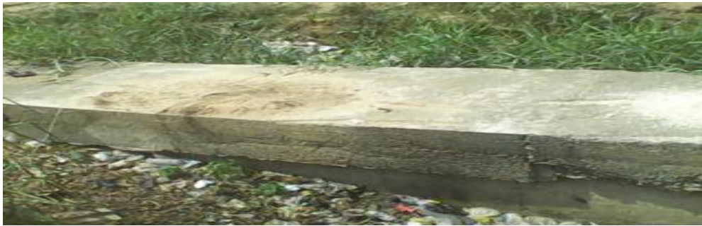
Plate 3. A section of the lined canal which convey water to the scheme
