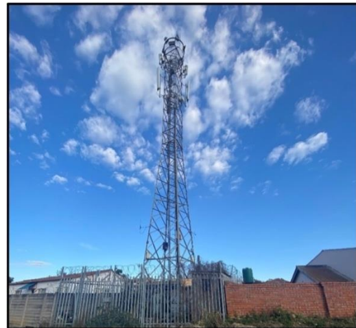
Fig. 13. Telecommunication towers built near houses
